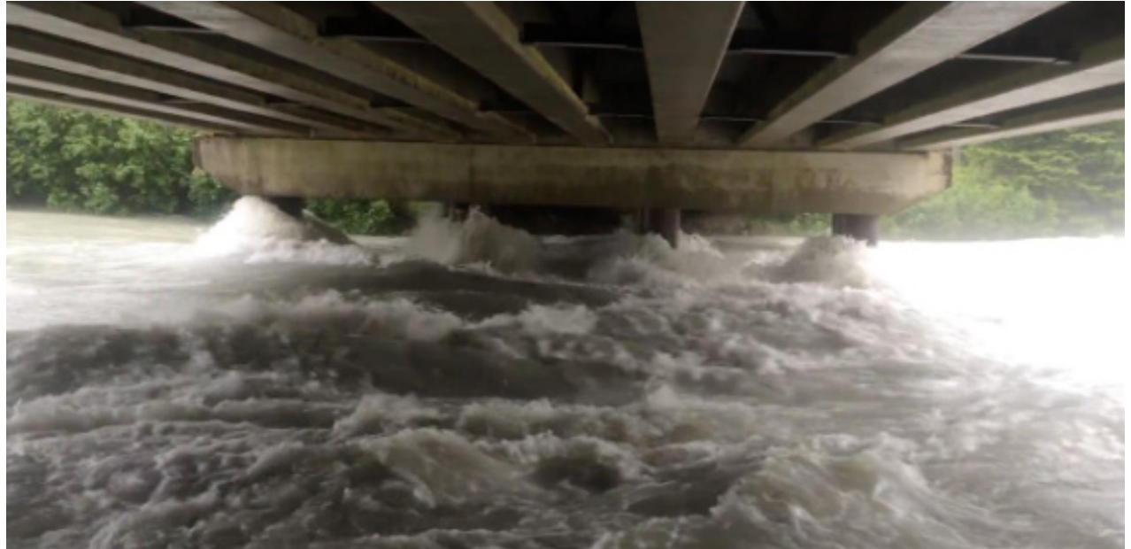
Figure G-6. Mendenhall River Bridge, Juneau, Jokulhlaup (Glacial Melting) Event 2016.
