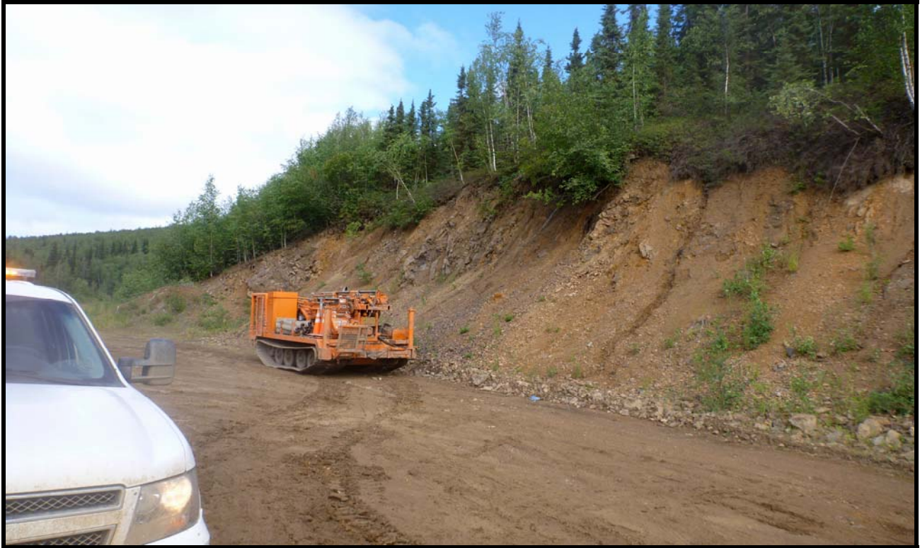
Figure 28: Existing Dalton Highway near station 510+00. Photo is looking north at east ditch with a highly weathered bedrock slope at the vehicle pullout.
