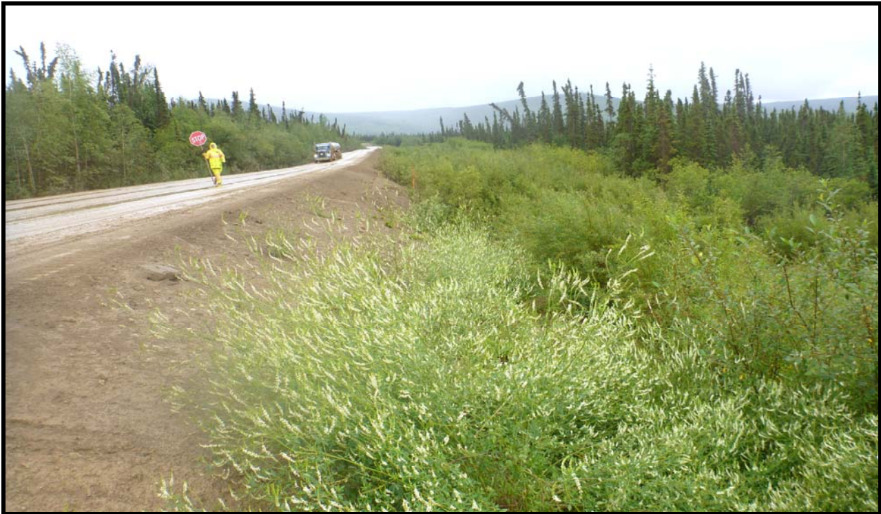
Figure 26: Existing Dalton Highway near station 458+50. Photo is looking southeast. The road has deep fills on the right and minor cut or fills on the left side. The ditch on the right is uneven ground with ponded water in some areas and drunken trees near those areas.
