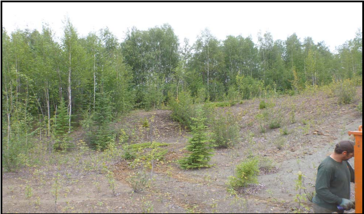
Figure 8: Proposed realignment near station 77+43. Photo is looking southwest at high ground composed mostly of highly weathered bedrock in a probable cut area. Photo is taken within a small material site excavation.
