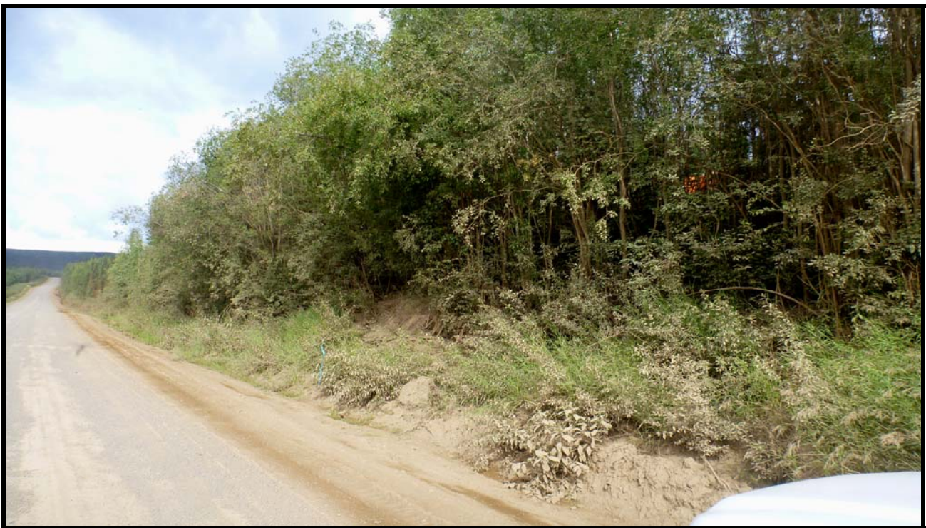
Figure 27: Existing Dalton Highway near station 467+00. Photo is looking northwest at north side ditch and side slopes at 7- to 10-feet higher in elevation than the road elevation. Drilling in the ditch at this location encountered highly ice-rich silts to 25-foot depth, indicating road widening in this area will cut into ice-rich side slopes.
