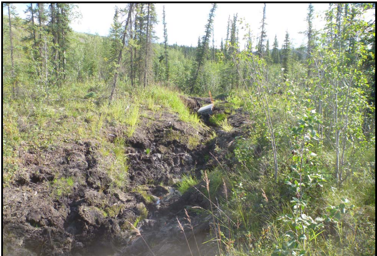
Figure 7: Existing utility easement near Rose Bud Creek and station 25+80. Photo is looking east with the Dalton Highway embankment to the left. The fiber optic excavation experienced approximately 3- to 4-feet of thaw settlement over a period of approximately two months in 2014.
