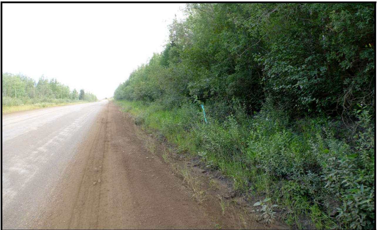
Figure 29: Existing Dalton Highway near station 537+00. Photo is looking to the north at east ditch side slopes. Test holes drilled on the slope encountered shallow thawed highly weathered bedrock.
